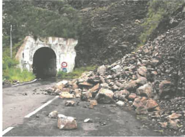
Éboulement RN5 – tunnel Peter Both (Cilaos) – Gamède 2007 © PPR Cilaos
